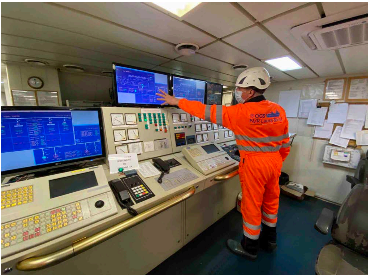
Controls of the engine room of R/V Laura Bassi.
